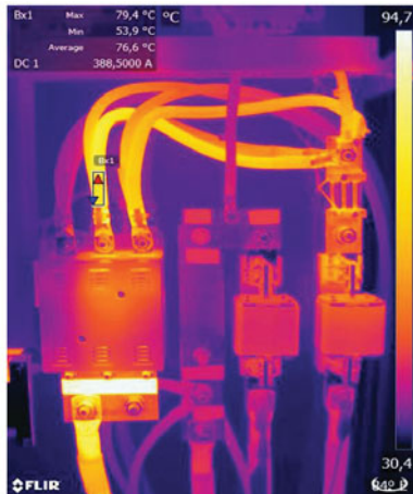
Thermal image in the electrical field for diagnosing a contactor with defective contacts
