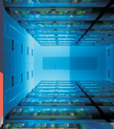
Energy Management Power Factor Correction BMS
