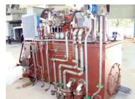
Hydraulic Power Packs
