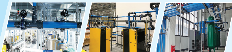
AIRpipe for Compressed airline system
