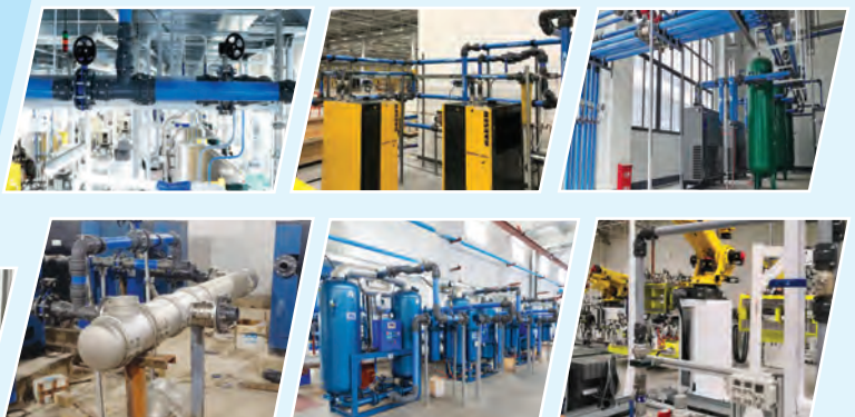
AIRpipe for Compressed airline system
