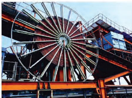
Cable Reeling Drums
