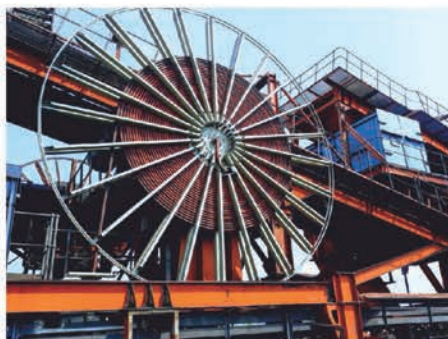
Cable Reeling Drums
