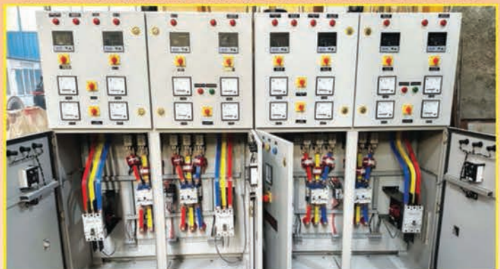
Furnace Control Panels
