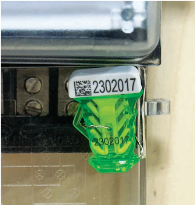
High security RevGuard smart security seal installed on meter.
