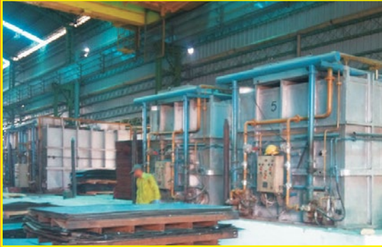
Gas Fired Rectangular Bell Furnaces
