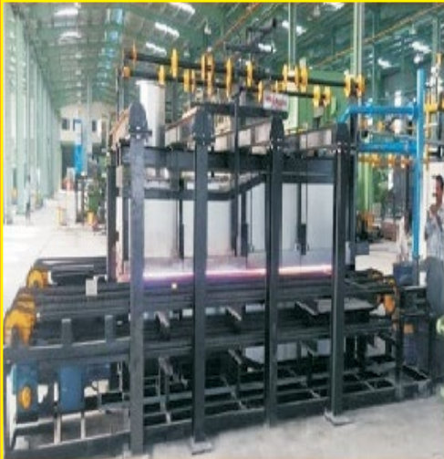
Conveyorised Heating Furnace
